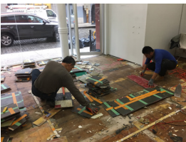
Wai Kong Lui and crew removing floor at PI, New York, 30 May 2017.
